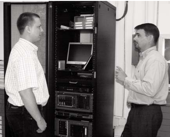
Right: Cliff Wilberding, Sales and Project Manager with NetBase Technologies, reviews system equipment with Rick Sullivan, Senior Design Technician and IT Director with Shows, Dearman and Waits. Shows, Dearman and Waits is a civil engineering firm that has been in business in the Hattiesburg area for more than 45 years.
